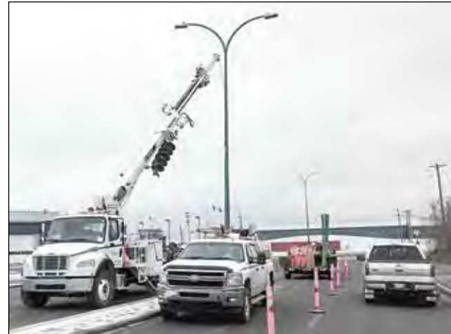
Northland Utilities crews work to replace streetlights along a median on Franklin Avenue. Re-lighting the street is one of the final steps of a two-year construction project.
